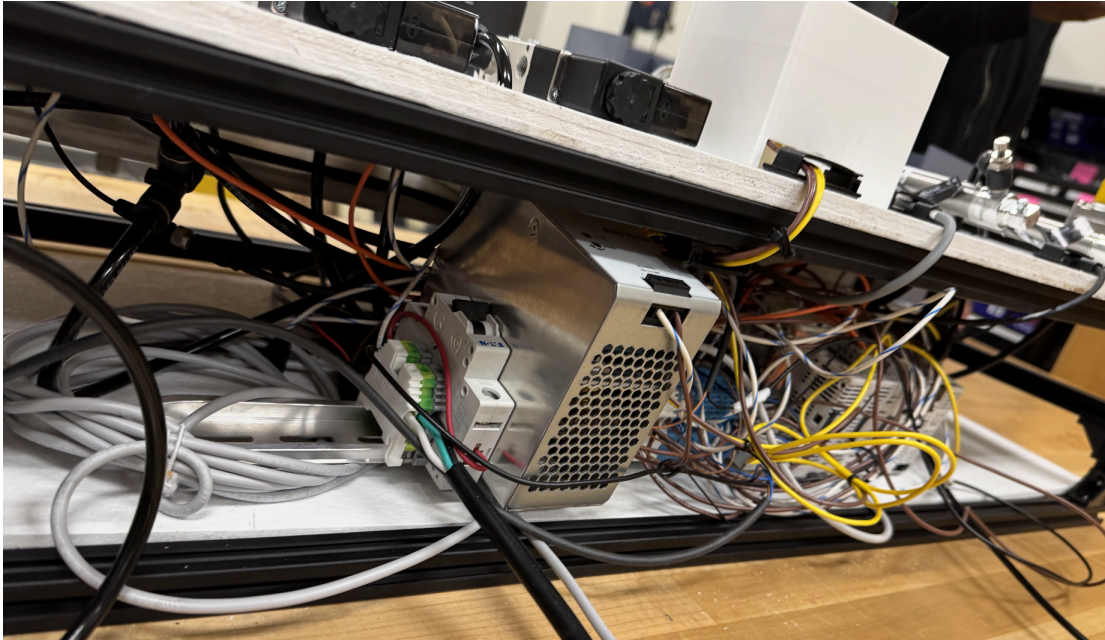
Figure 5: Final Wiring, Cables, and Tubing Orientation Underneath the Platform
